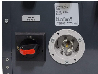
Figure 10-1 Disconnect switch and power supply connection
