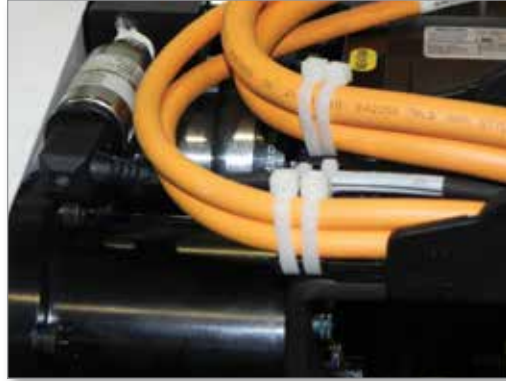
Figure 7-2 Cables held with wire ties
