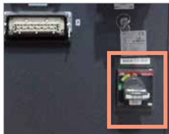
Figure 6-1 E-Multi main power switch
