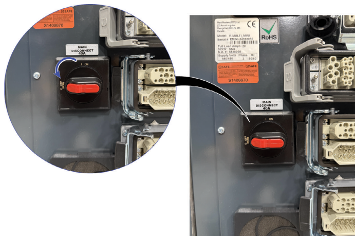
Figure 7-1 Main power switch
