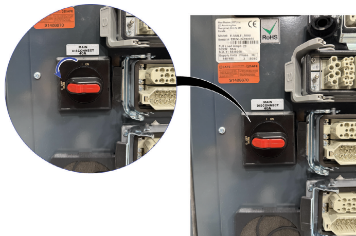
Figure 7-1 Main power switch
