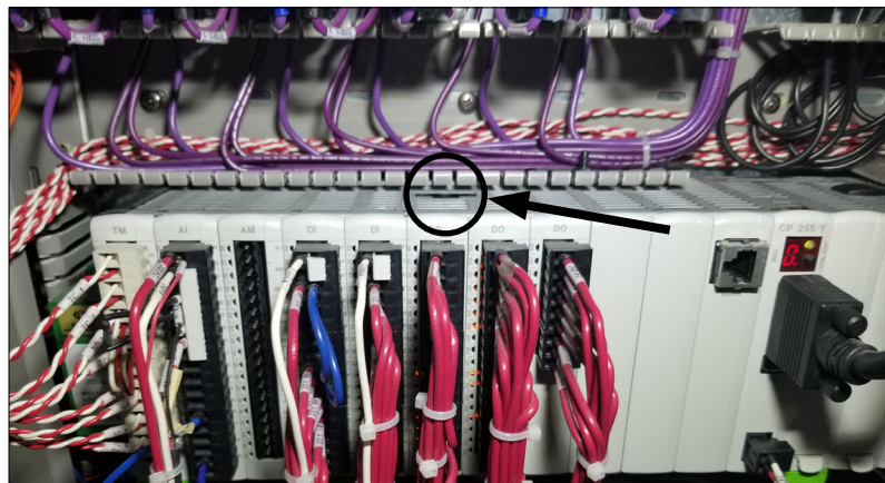
Figure 9-4 Location of the CMOS battery tray (older cabinets)
