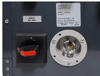
Figure 10-1 Disconnect switch and power supply connection
